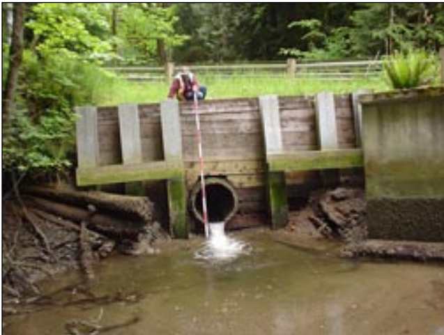
An undersized culvert partially blocks fish access to one mile of stream on The Evergreen State College campus in Olympia, WA.
