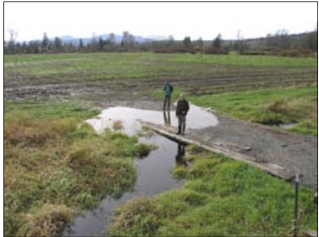
A failing culvert and road crossing at Indian Creek.
