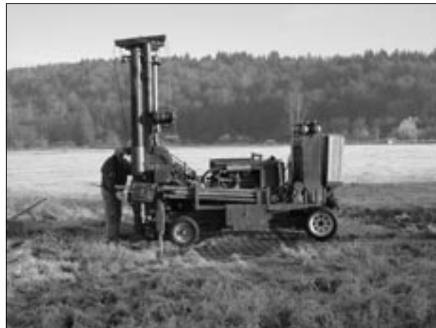
Sub-contractors from Cascade Drilling Inc. install a groundwater monitoring well in Cherry Valley.
